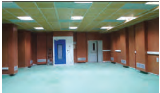
Clean room in building No: 5206
